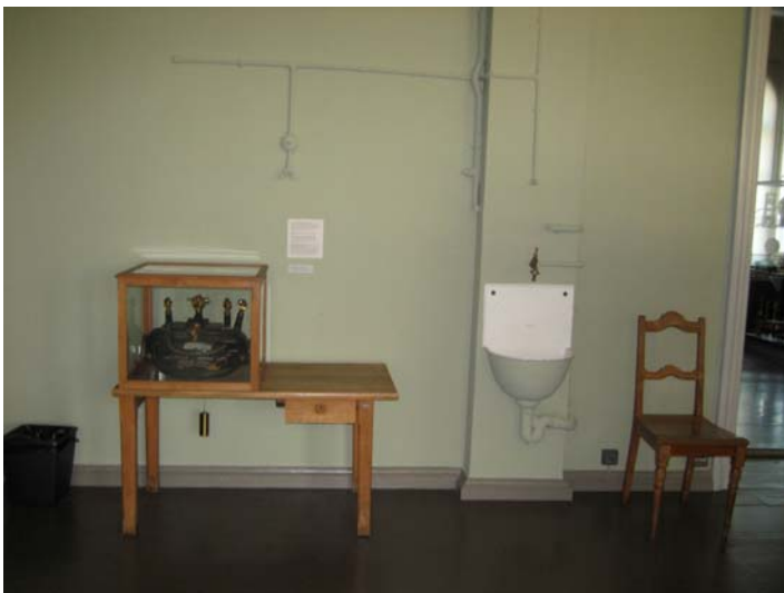
Fig. 3 - Original gas pipes and sinks were left as evidence of the previous history of the building. Photo K. Heinämies, Helsinki University Museum
