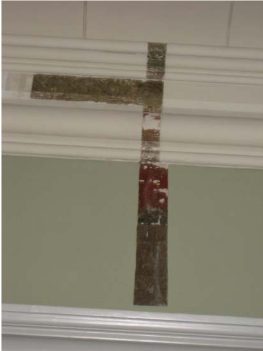
Fig. 2 - The previous layers of paint uncovered before the restoration. Photo K. Heinämies, Helsinki University Museum
