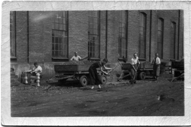
Fig. 14. After-hours volunteer work to build an employee rest area at MAN, Augsburg. Private photo, 1935. Source: Historisches Archiv der MAN, Augsburg, file group 2.2.3/19.
